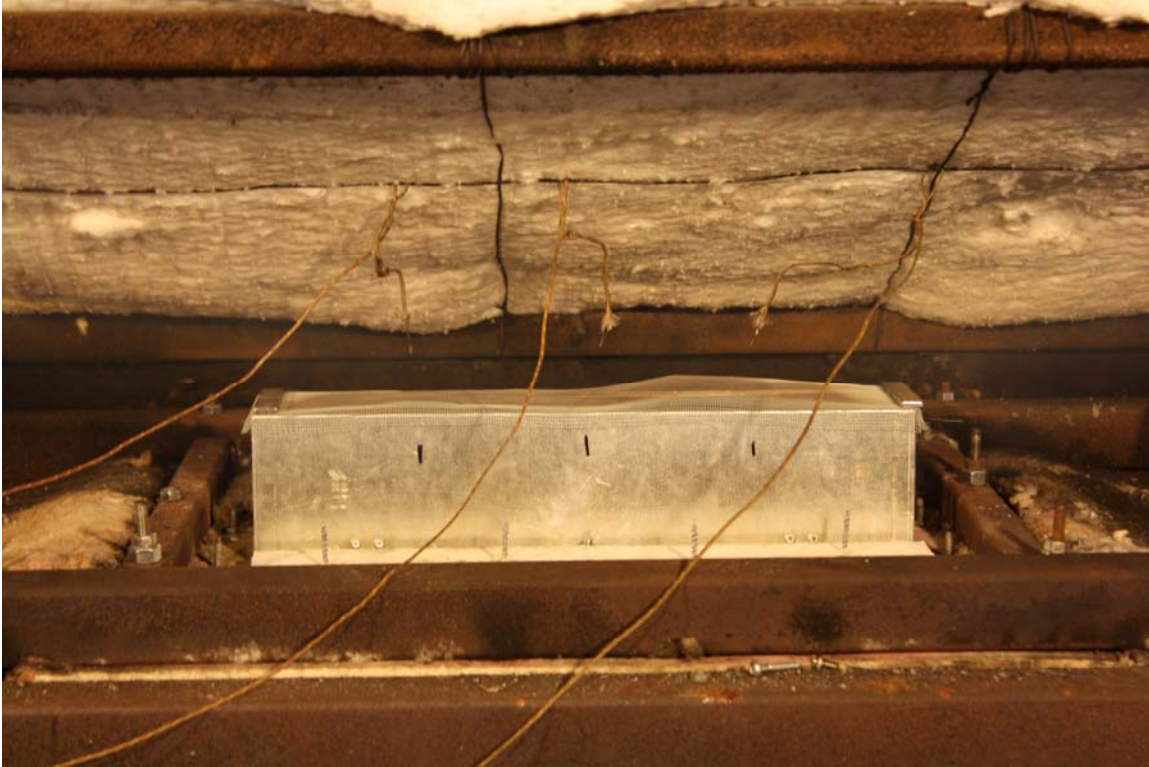
Vent exit side during flame intrusion exposure
